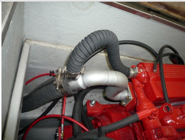
Engine exhaust injection point
