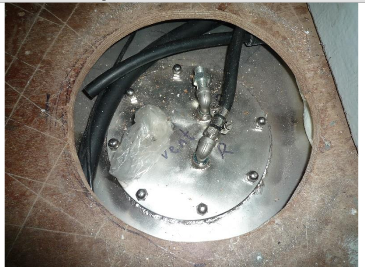
Fuel tank not yet fully connected
