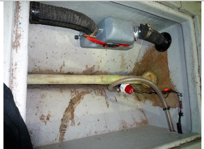
New grp propeller shaft tube and non secured electric bilge pump. This area is awaiting additional ballast before the pump is finally located. The unsupported length of prop shaft just falls within the acceptable maximum length.
