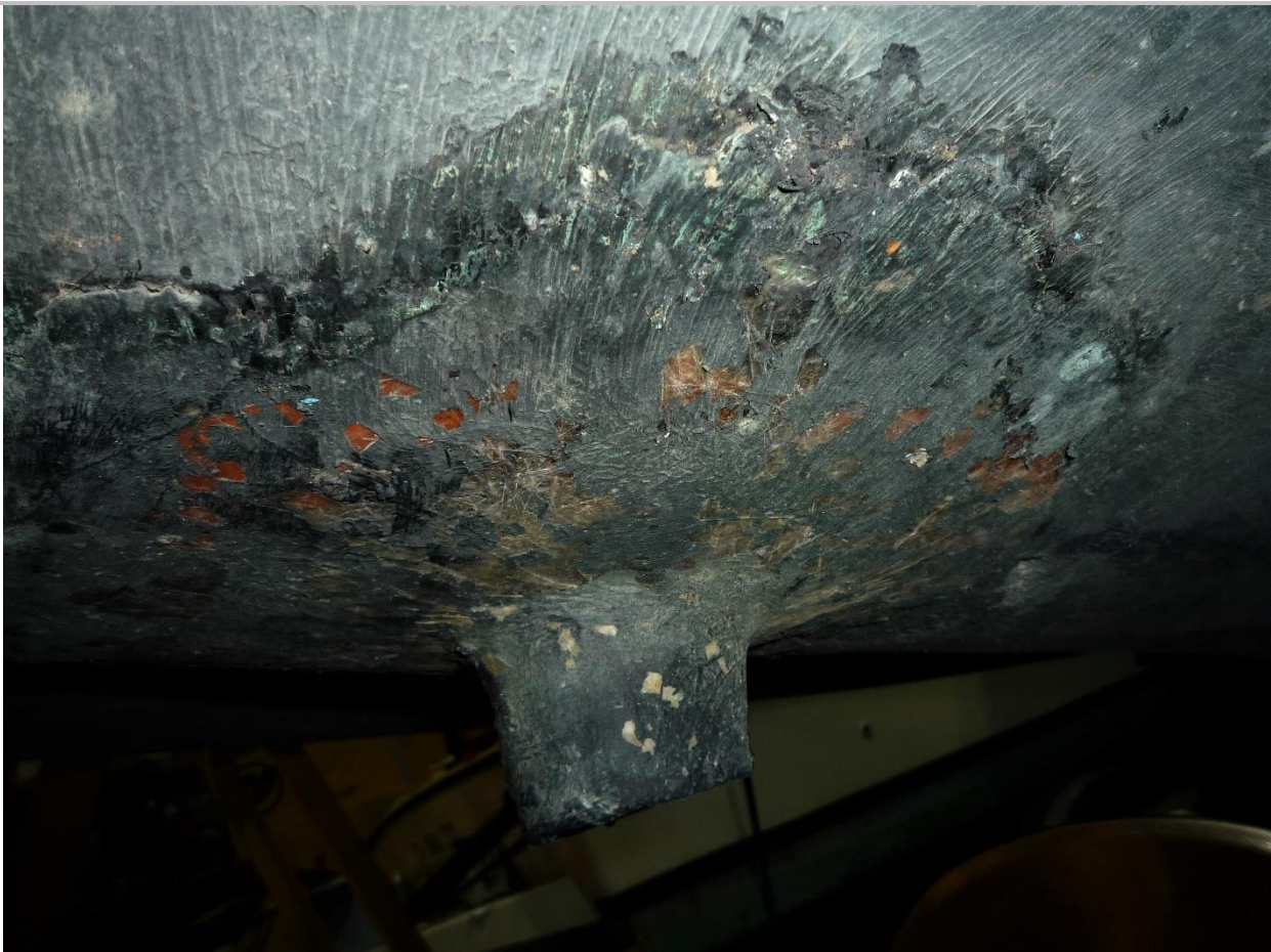
This photograph shows the failing laminates around the external rudder tube location
