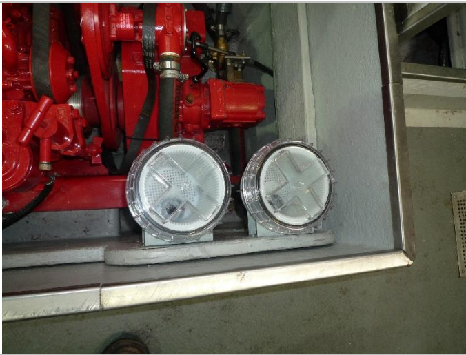
Engine water strainers. These are new. It is likely these are not approved strainers.
