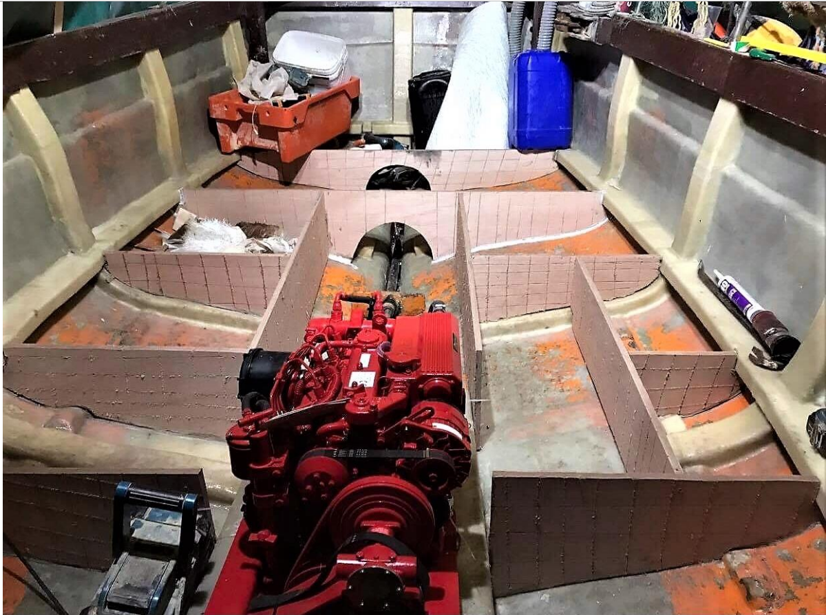
Applicant supplied photo of the deck construction in build. From this it would appear that the individual compartments are probably less than 1 cu.mtr. No major athwartships floors but considerable stiffening in the lower bilges
