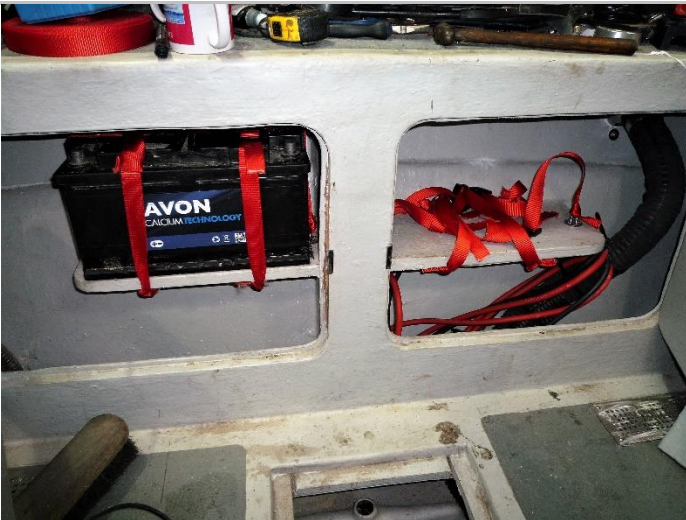
Battery storage under aft deck
